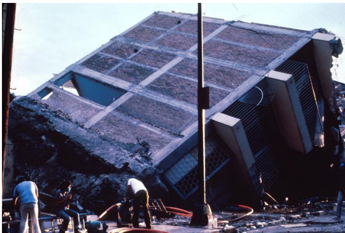
Figure 22: Building collapse due to liquefaction of soil sediments. Image courtesy of Wikispaces.com ( http://earthscienceinmaine.wikispaces.com/7.4+Staying+Safe+in+Earthquakes )
